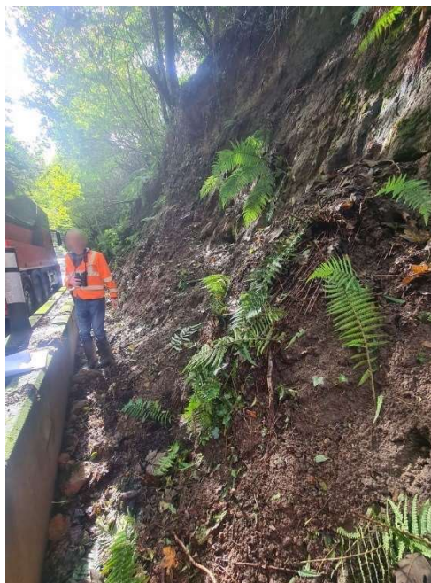
Figure 12 – October 2023 landslide on the West Site
