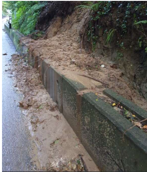
Figure 11 – October 2021 landslide from the East Site
