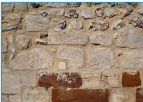
Swanage brick produced using local Wealdon clay, and a wall containing an unusual mix of local flint, limestone and heathstone.
