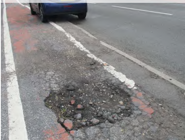
Figure 1.7: Poor road surface conditions within a cycle lane
