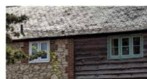
Casement windows (uPvc)
