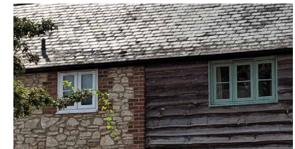
Casement windows (uPvc)
