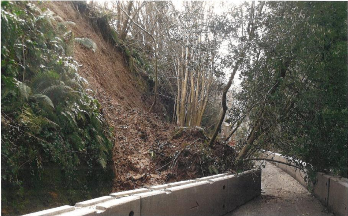
Figure 1: Landslip – viewing South
