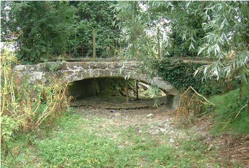
Footbridge over the River Winterborne near its confluence with the River Stour at Sturminster Marshall
