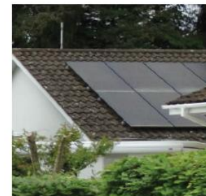
Roof solar panelling.
