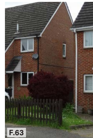
Figure 63: Example of gutters which are inconsistent in colour between neighbouring dwellings.
