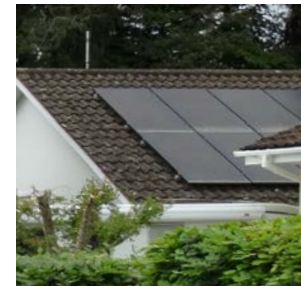
Roof solar panelling.
