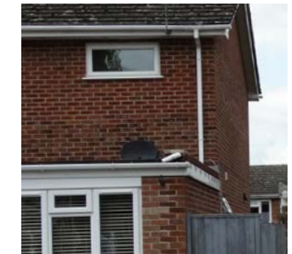
Satellite dish pushed back from the street scene.
