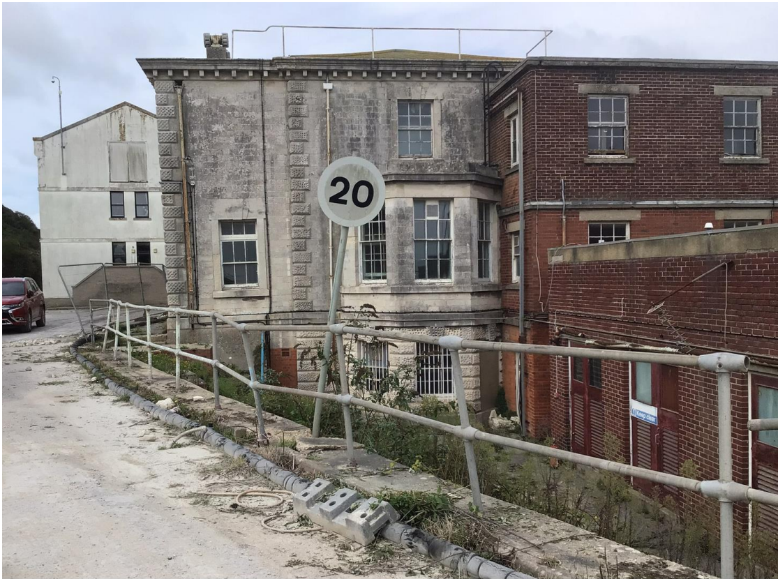
Dockyard Offices, projecting bay with modern extension, the projecting bay is altered but not fully obscured
