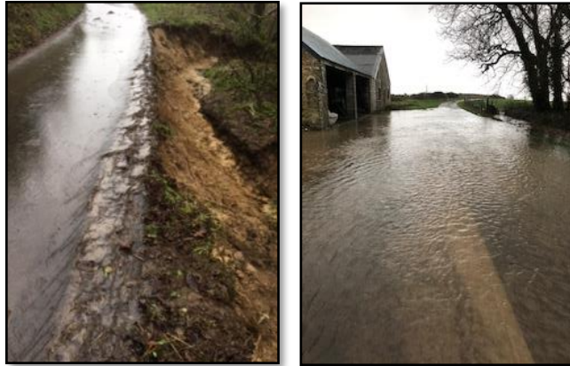
Photo 3 – Bank collapse and flooding at Portesham Farm
